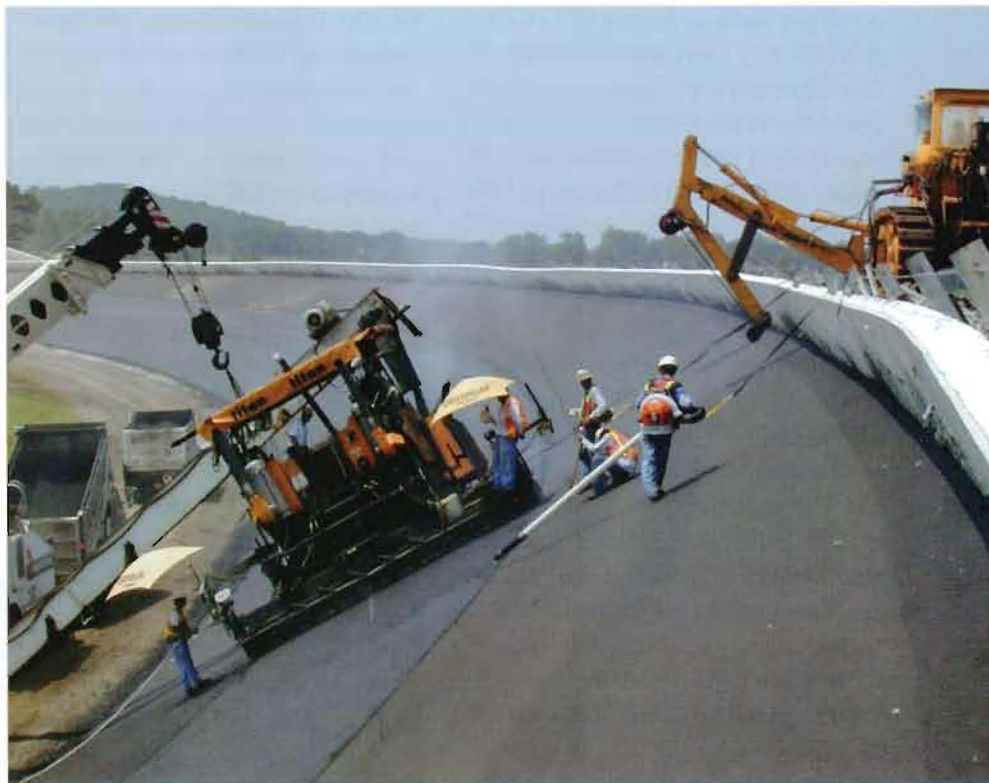
The north and south turns have a maximum banking of 33 degrees, which meant the paving crew needed specialized equipment to do their jobs properly.
