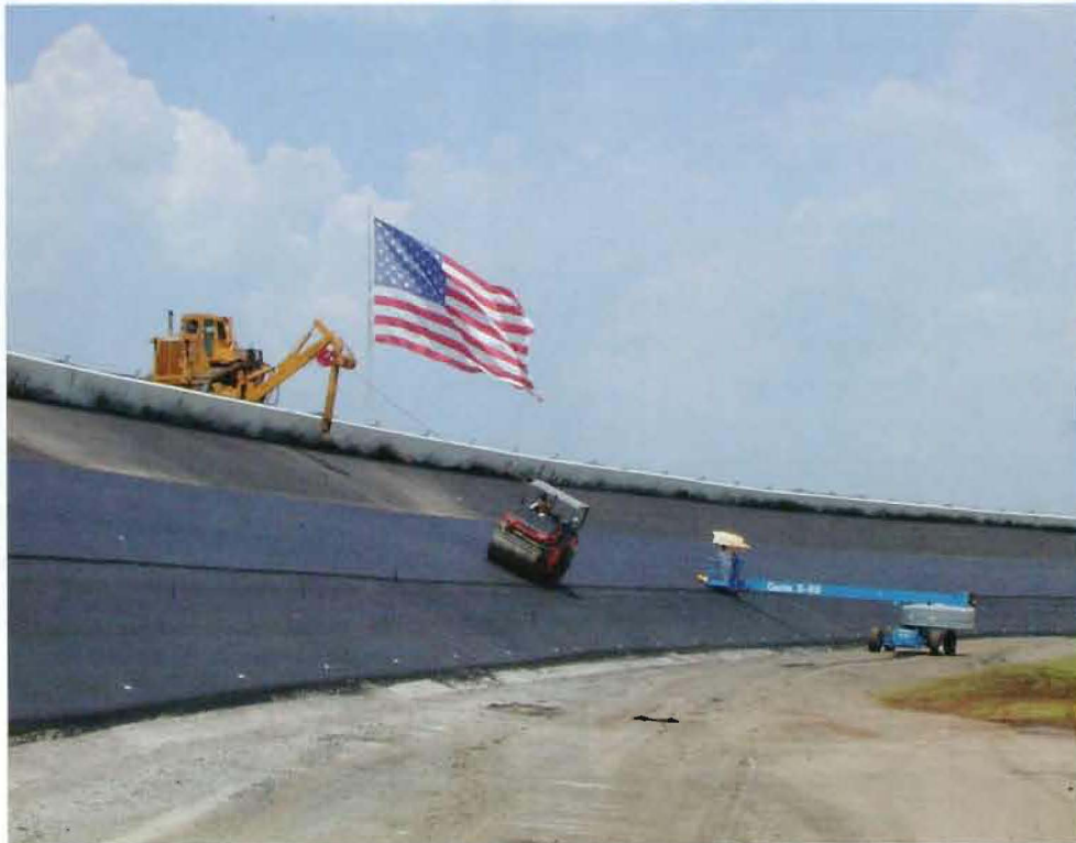
The mill and overlay project at the speedway required some 50,000 tons of asphalt and a total of five different mixes. The project emphasized smoothness, durability and proper drainage for the track.
