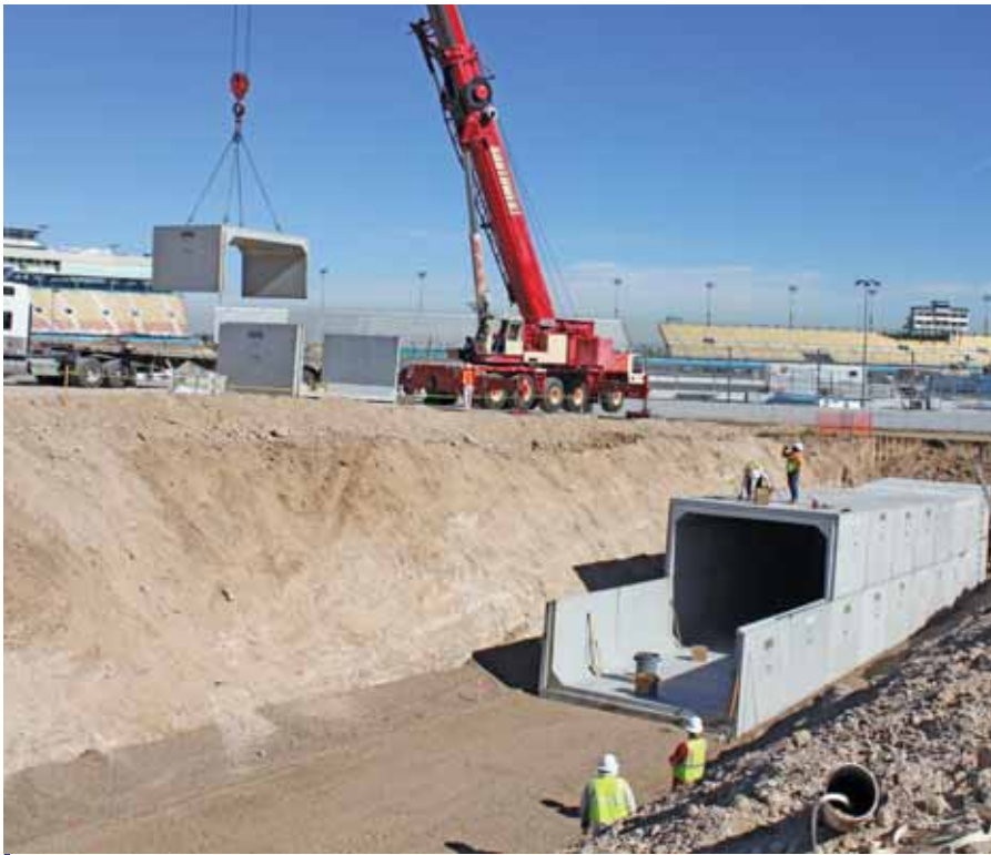
ISC has built two new pedestrian tunnels under the Phoenix track, one under Turn 1 and one under Turn 2. They open-cut the track and then backfilled around the tunnel.
