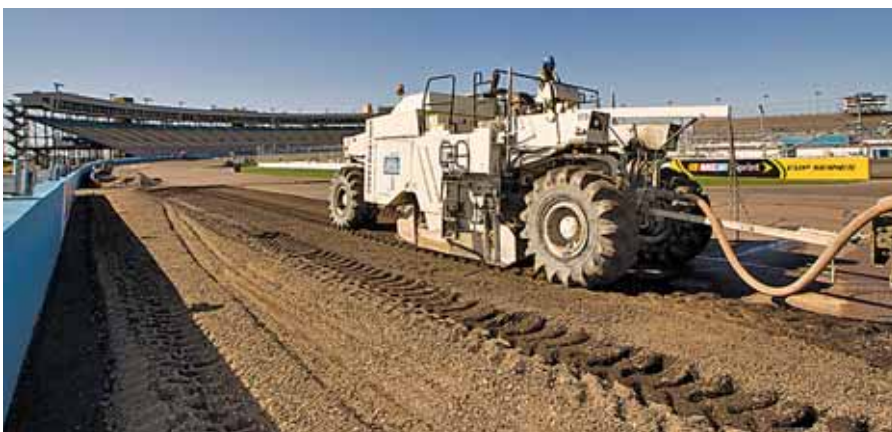
The final details of the Phoenix asphalt mix are not yet settled, but Braniff said the pavement would consist of a 4-in. aggregate base course of crushed rock. Over that will be a 2-in. asphalt base course, a 1.5-in. leveling course and a 1.5-in. wearing course.
