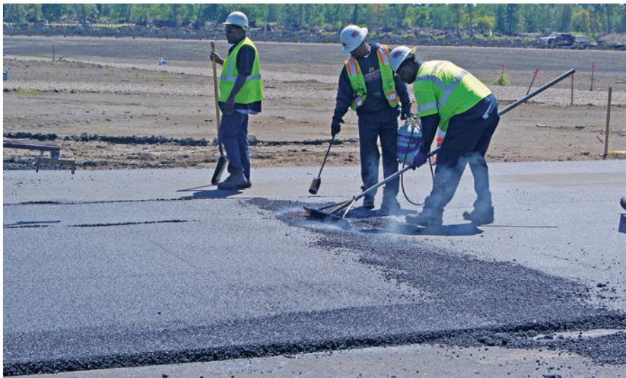
Workers heat and smooth a transverse joint by hand. The asphalt mix used at NOLA is a 5-in. pavement, put down in three lifts. The base course is 2 in. of a conventional Louisiana DOT mix, with 12.5-mm aggregate size and a 67-22 or 64-22 binder.
