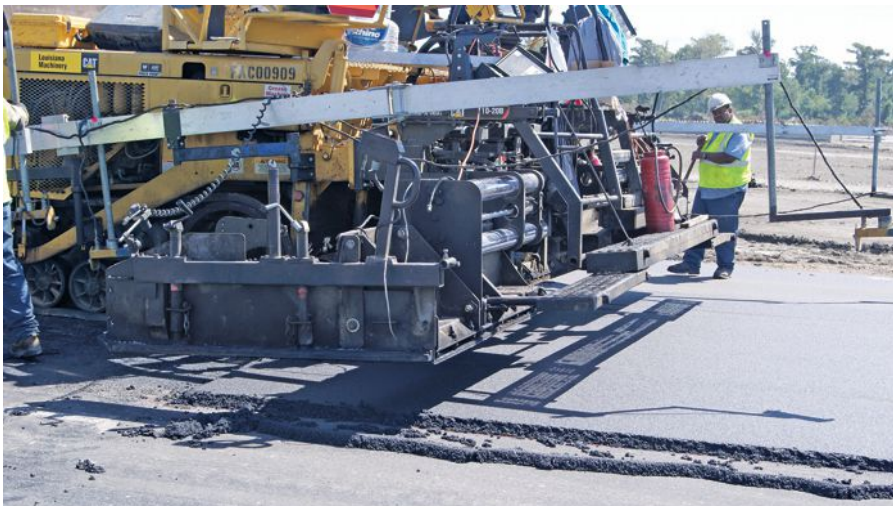
Above: The paving crew attempts to place the screed exactly where it was when it encountered a problem getting around a sharp corner.
