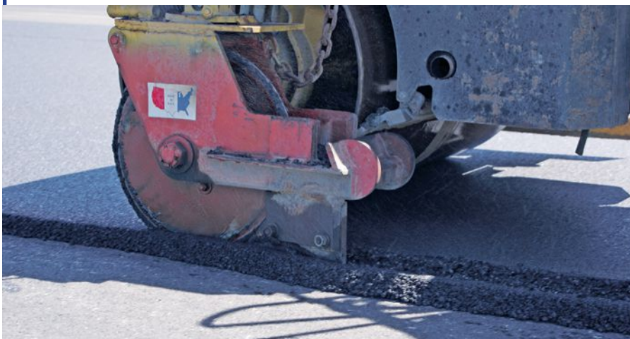
Below: The longitudinal joint down the middle of the NOLA track is cut by a special roller with a cutting wheel following behind the other rollers.
