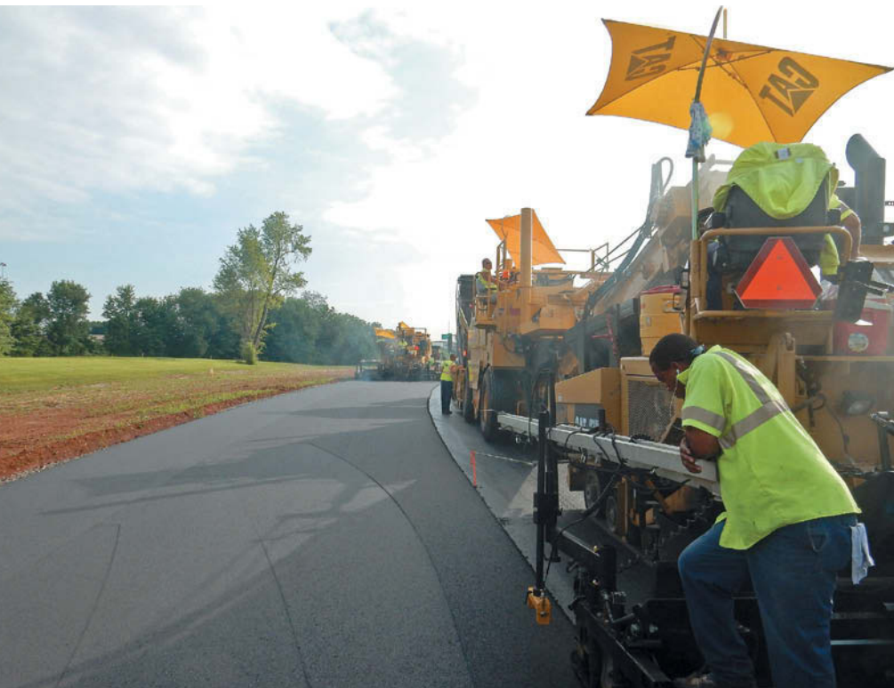
Echelon paving of the specialized surface course using two pavers at once eliminated cold longitudinal joints between pulls at the NCM Motorsports track. Photo credit: Scotty's Contracting & Stone LLC
