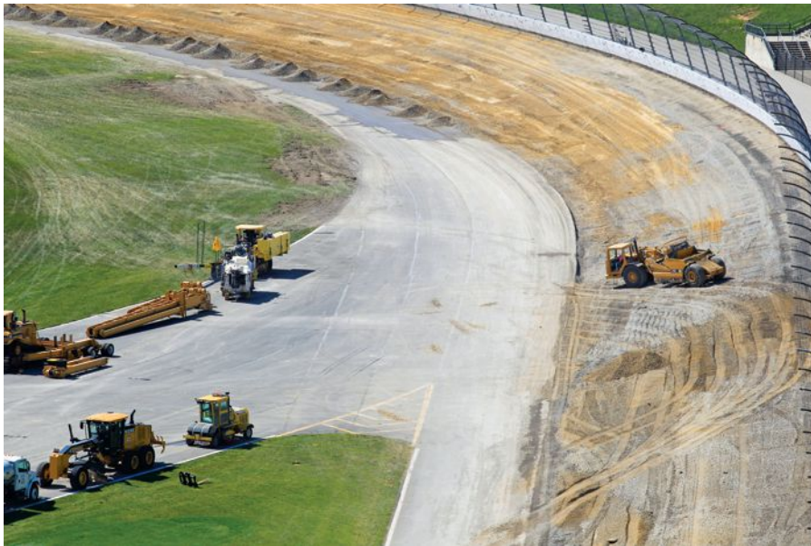
Caterpillar D6T and D6R dozers were cutting as much as 2 ft deep into material to establish the new slopes on the turns. The original plan was to push the bulk of dirt upward before a Caterpillar motor grader smooths out the surface.
