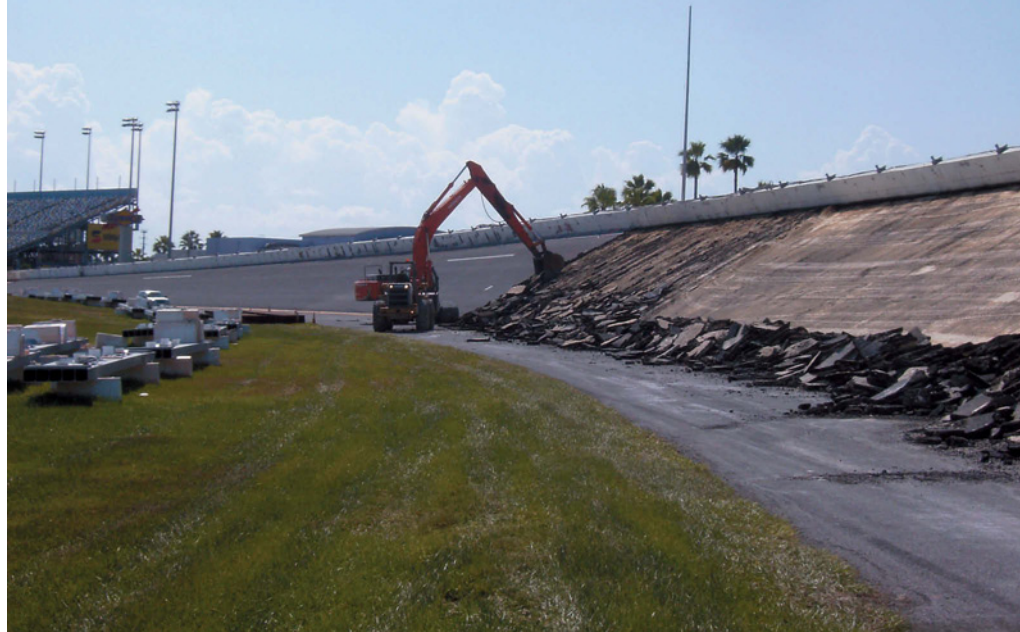
2010: A tracked excavator was used for demolition in the turns. Photo by Brian Prowell.
