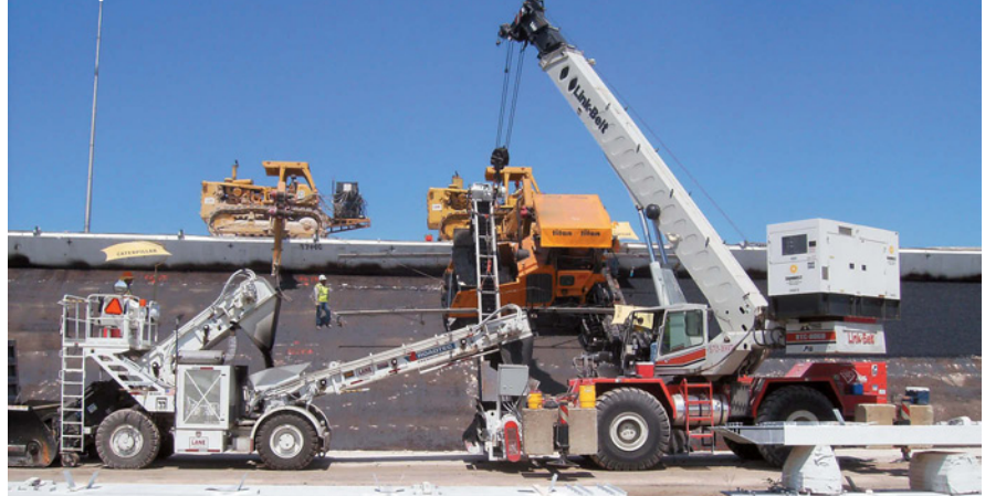
2010: It takes a lot of people and a lot of iron to pave from the top down. Photo by Brian Prowell.
