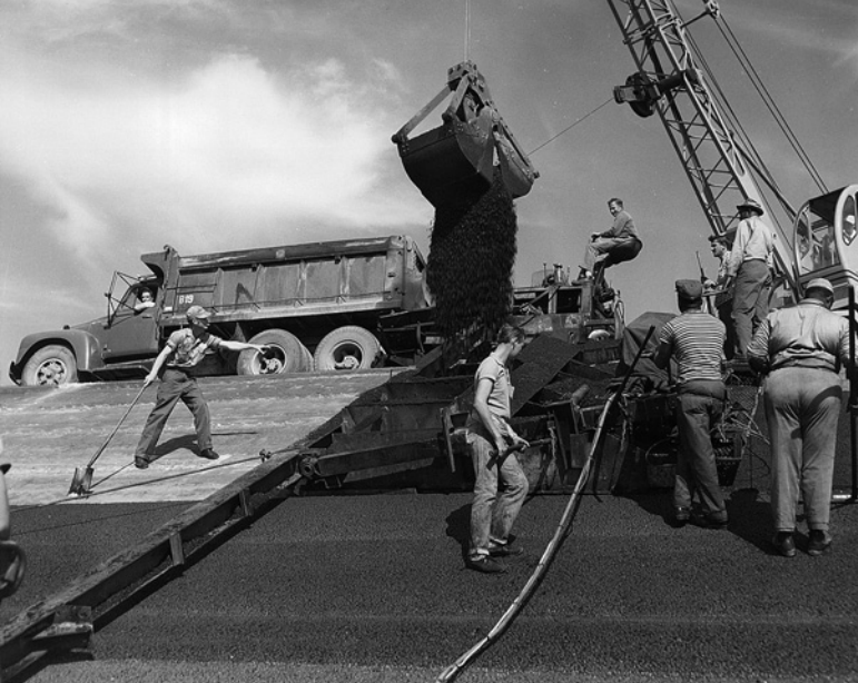
1958: In this photo snapped during the original construction of Daytona, a crew waits for pavement material to drop onto the surface of the track.
