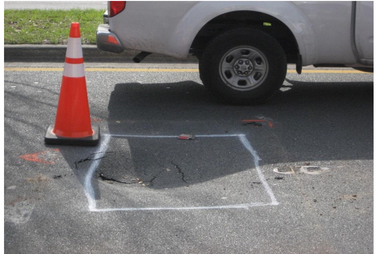
Pavement depression after steel plate was removed
