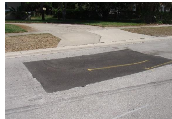
Pavement Depressions/High Moisture
